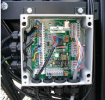
Figure 14 Terminals for connecting the sensors
